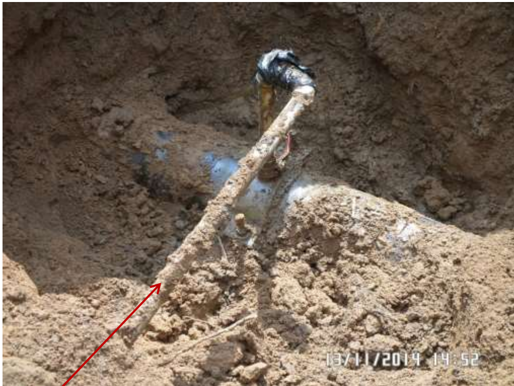
Close-up: Illegal fitting on 8" Nkpoku-Bomu Pipeline at Umuechem. Picture was taken during Joint Investigation of 13 th November 2014.
