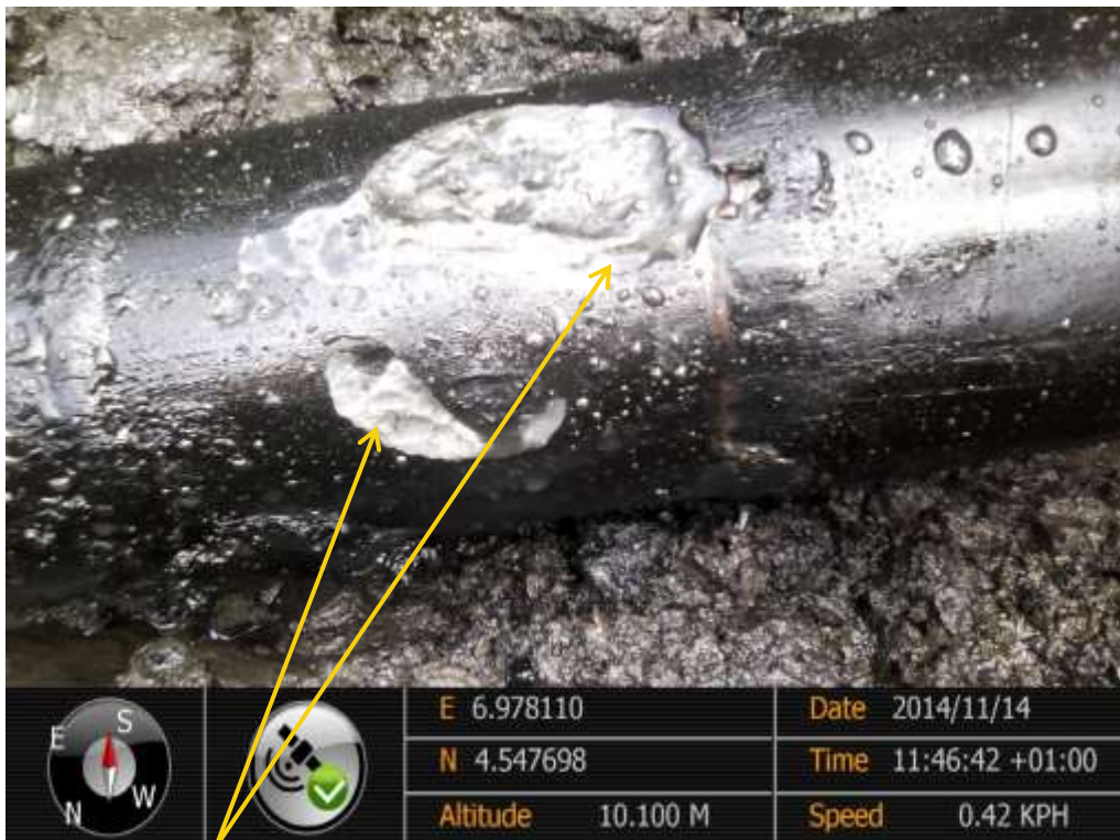
Close-up: Spill due to corrosion on Cawthorne Channel3 Well4LS Flowline at Sand Sand. Picture was taken during Joint Investigation of 14 th November 2014.
