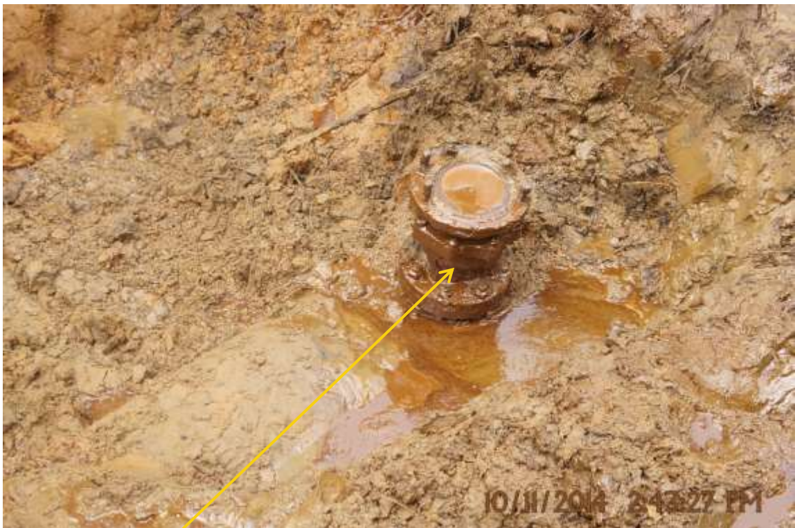
Close-up: Illegal fitting on 20" Otumara – Escravos Pipeline at Ogidigben. Picture was taken during Joint Investigation of 10 th November 2014.
