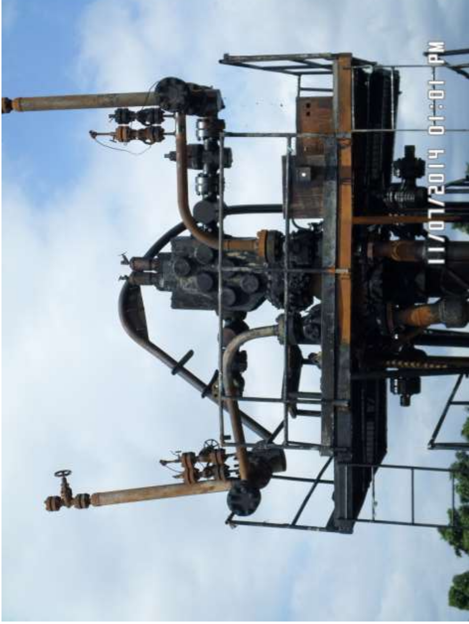
AKASO WELL3 WELLHEAD AT ILOMATURU
