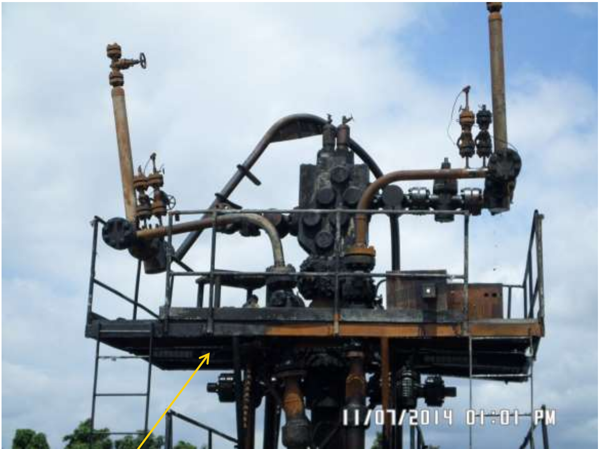
Close-up: Fire damage on Akaso Well3 Wellhead at Ilomaturu. Picture was taken during Joint Investigation of 7 th November 2014.
