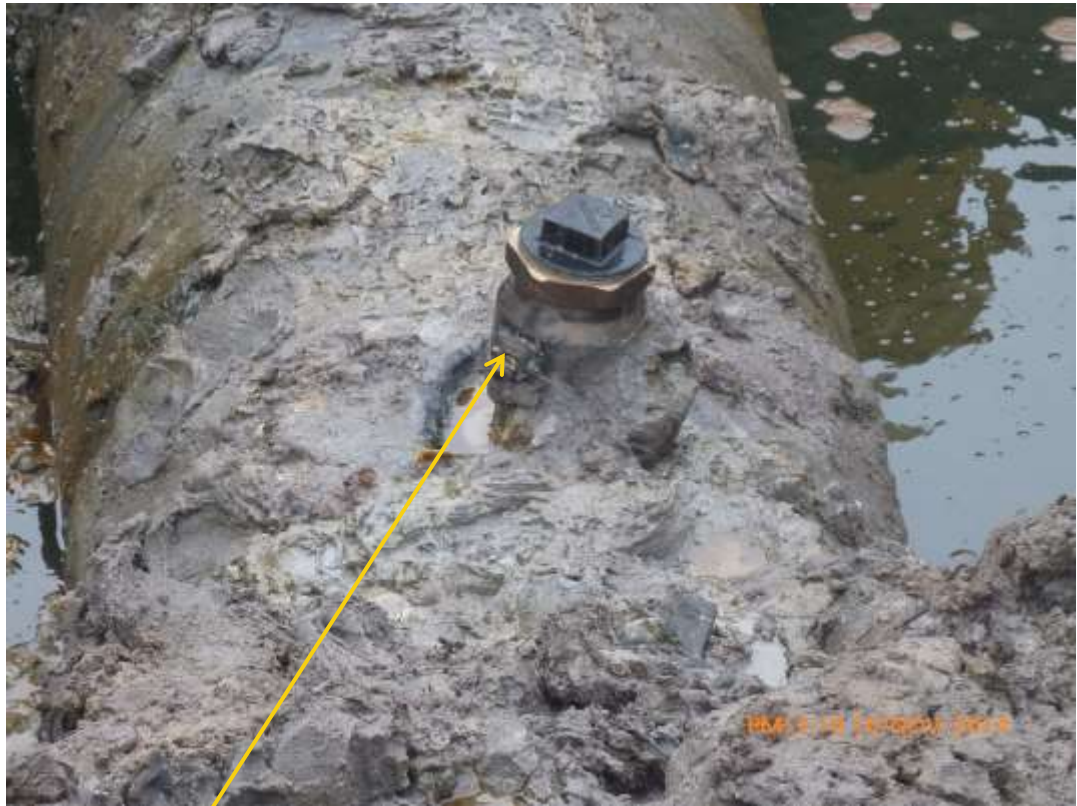
Close-up: Illegal fitting on 28" Bomu-Bonny Pipeline at Bodo City. Picture was taken during Joint Investigation of 9 th November 2014.
