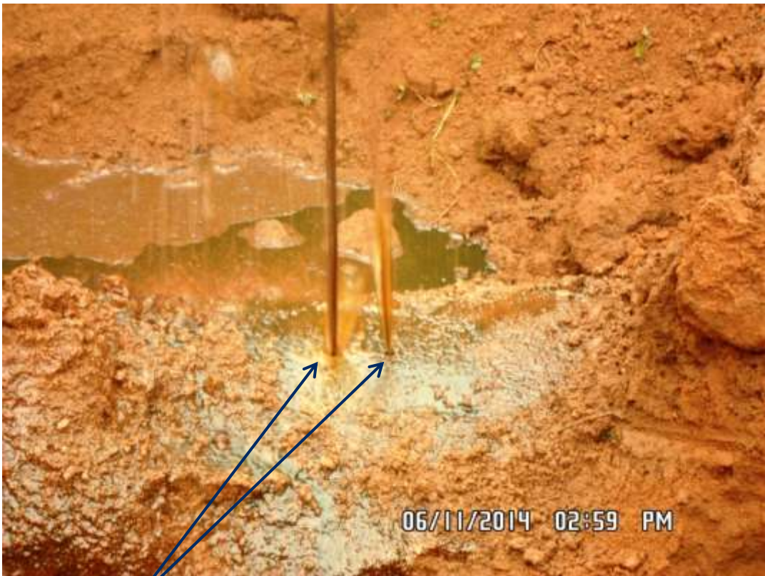
Close-up: Drilled holes on 28" Nkpoku-Bomu Pipeline at Norkpo. Picture was taken during Joint Investigation of 6 th November 2014.
