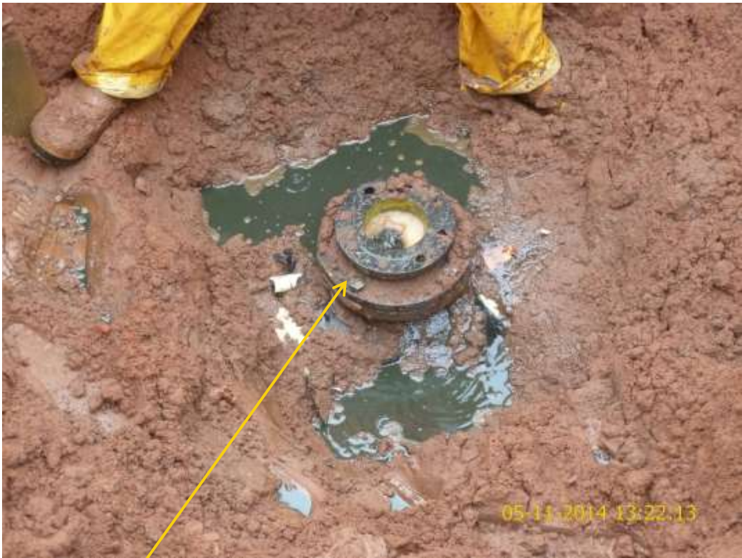
Close-up: Illegal fitting on 16" Egbema-Assa Trans Niger Pipeline at Umudike. Picture was taken during Joint Investigation of 5 th November 2014.
