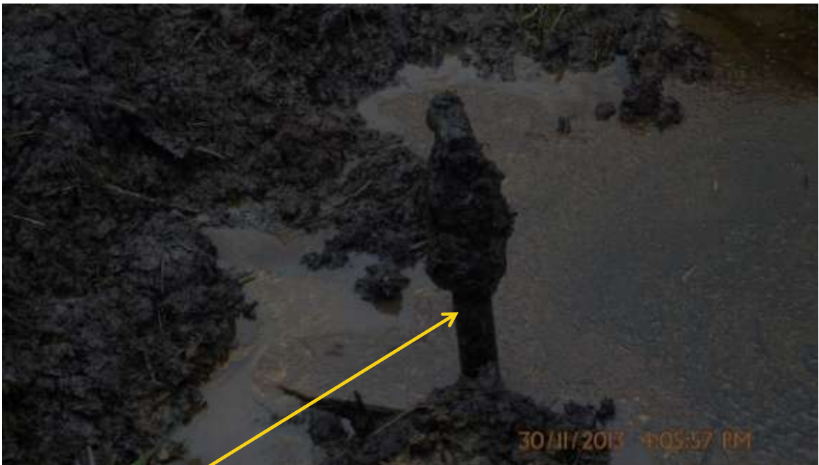
Close-up: Illegal fitting on 20" Opukushi-Brass Creek Trunkline at Tamogbene. Picture was taken during Joint Investigation of 30 th November 2013.
