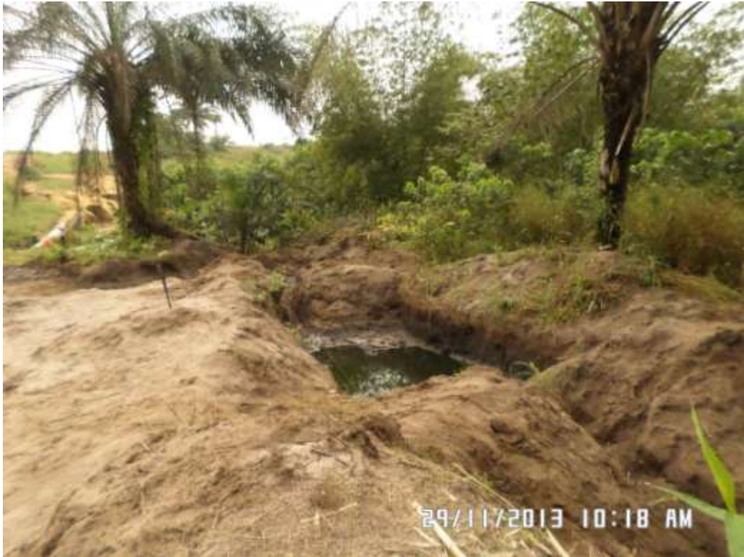
Overview: Part of spill impact on 28" Nkpoku-Bomu Pipeline at Gio. Picture was taken during Joint Investigation of 29th November 2013.
