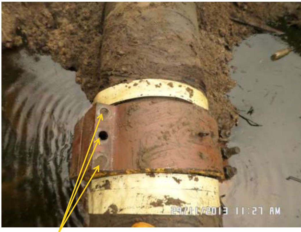
Close-up: Nuts removed from clamp on 28" Nkpoku-Bomu Pipeline at Gio. Picture was taken during Joint Investigation of 29th November 2013.
