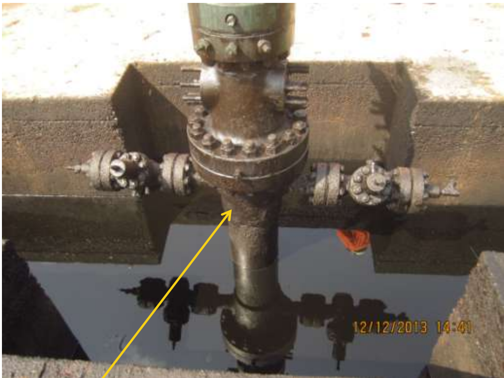
Close-up: Failed valve on Elenwo Well9LS Wellhead at Elenwo. Picture was taken during Joint Investigation of 12th December 2013.
