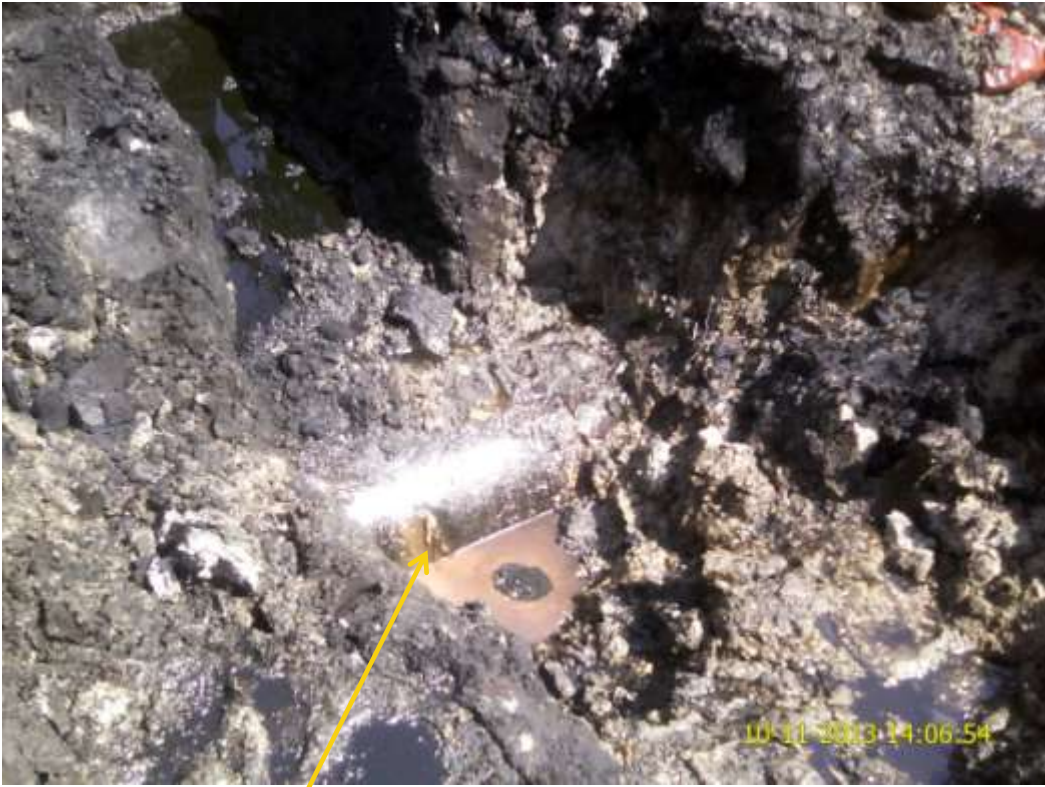
Close-up: Hacksaw cut on 24" Bomu-Bonny Pipeline at Kpor. Picture was taken during Joint Investigation of 10 th November 2013.
