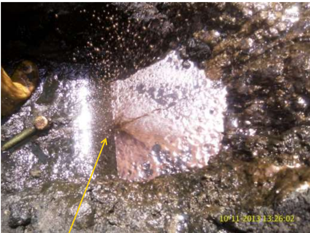
Close-up: Hacksaw cut on 24" Bomu-Bonny Pipeline at Kpor. Picture was taken during Joint Investigation of 10 th November 2013.
