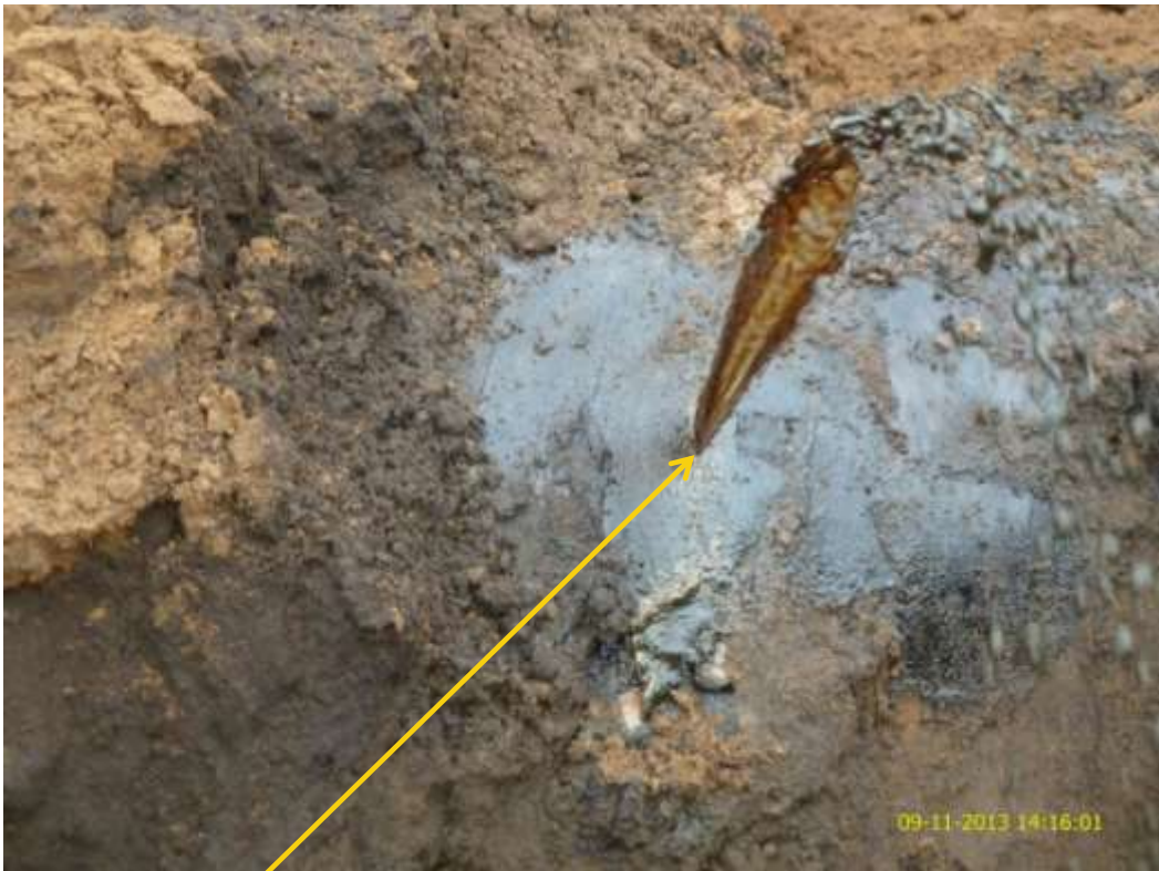
Close-up: Hacksaw cut on 28" Bomu-Bonny Trans Niger Pipeline at Bodo City. Picture was taken during Joint Investigation of 9 th November 2013.
