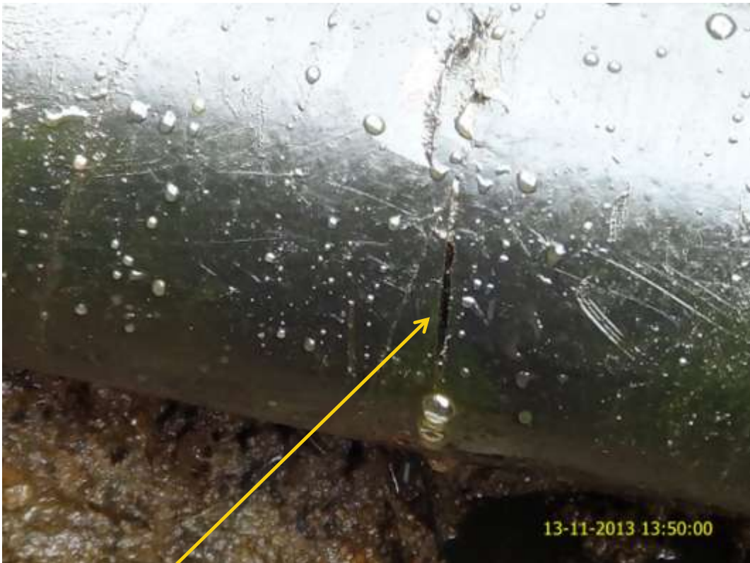
Close-up: Hacksaw cut on ImoRiver Well21L Flowline at Igiriukwu/Isietitioha. Picture was taken during Joint Investigation of 13 th November 2013.
