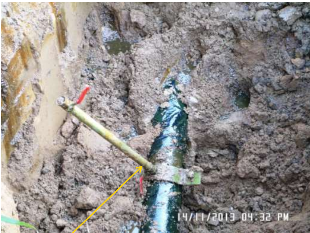
Close-up: Illegal fitting on 6" Obigbo North – Ogale Pipeline at Ogale. Picture was taken during Joint Investigation of 14th November 2013.
