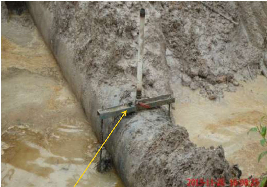
Close-up: Illegal fitting on 24" Nkpoku - Bomu Trans Niger Pipeline at Eteo. Picture was taken during Joint Investigation of 20th November 2013.
