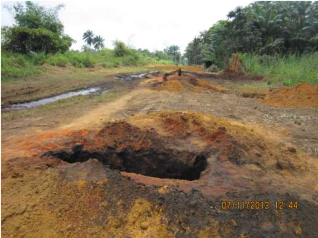
Overview: Part of spill/fire impact on 24" Bomu – Nkpoku Pipeline at Kpите. Picture was taken during Joint Investigation of 7th November 2013.
