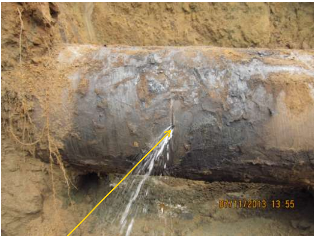
Close-up: Hacksaw cut on 24" Bomu - Nkpoku Pipeline at Kpите. Picture was taken during Joint Investigation of 7th November 2013.
