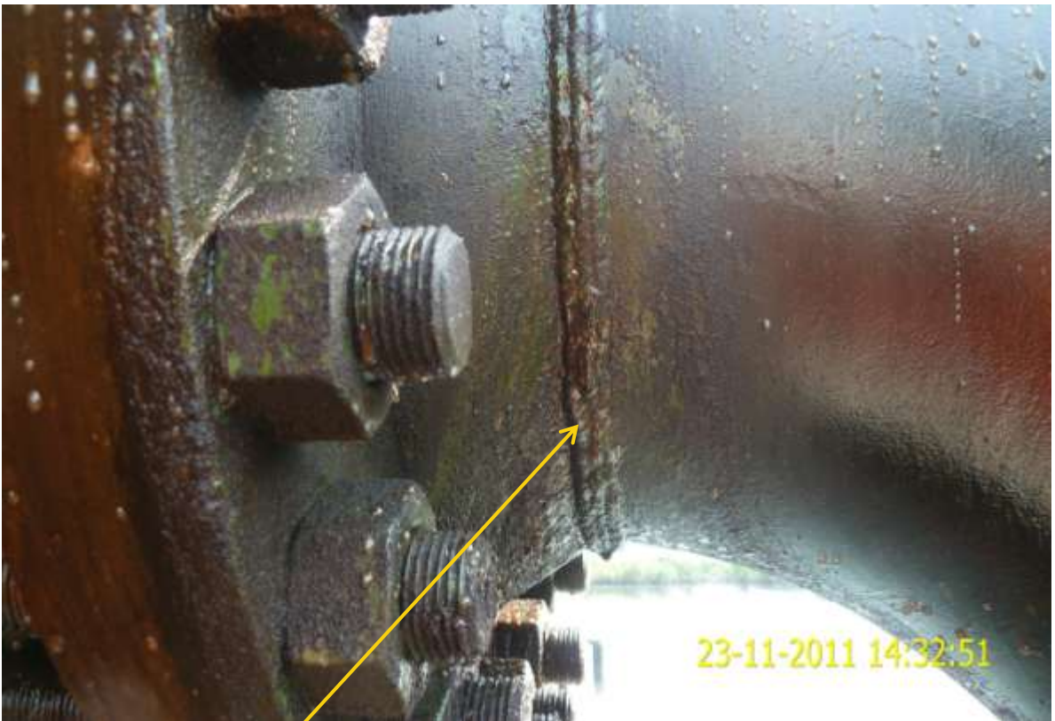
Close-up: Spill due to failed weld on 12" Cawthorne Channel pipeline riser at Ilomaturu. Picture was taken during Joint Investigation of 23 rd November, 2011.
