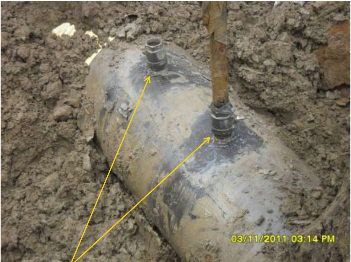
Close-up: Illegal fittings on 24" Npoku-Bomu pipeline at Biara. Picture was taken during Joint Investigation of 3 rd November, 2011.
