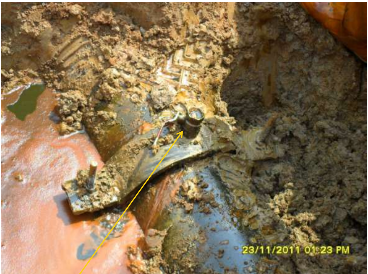
Close-up: Illegal fitting on 12" ImoRiver2-Ebubu pipeline at Odagwa. Picture was taken during Joint Investigation of 23 rd November, 2011.
