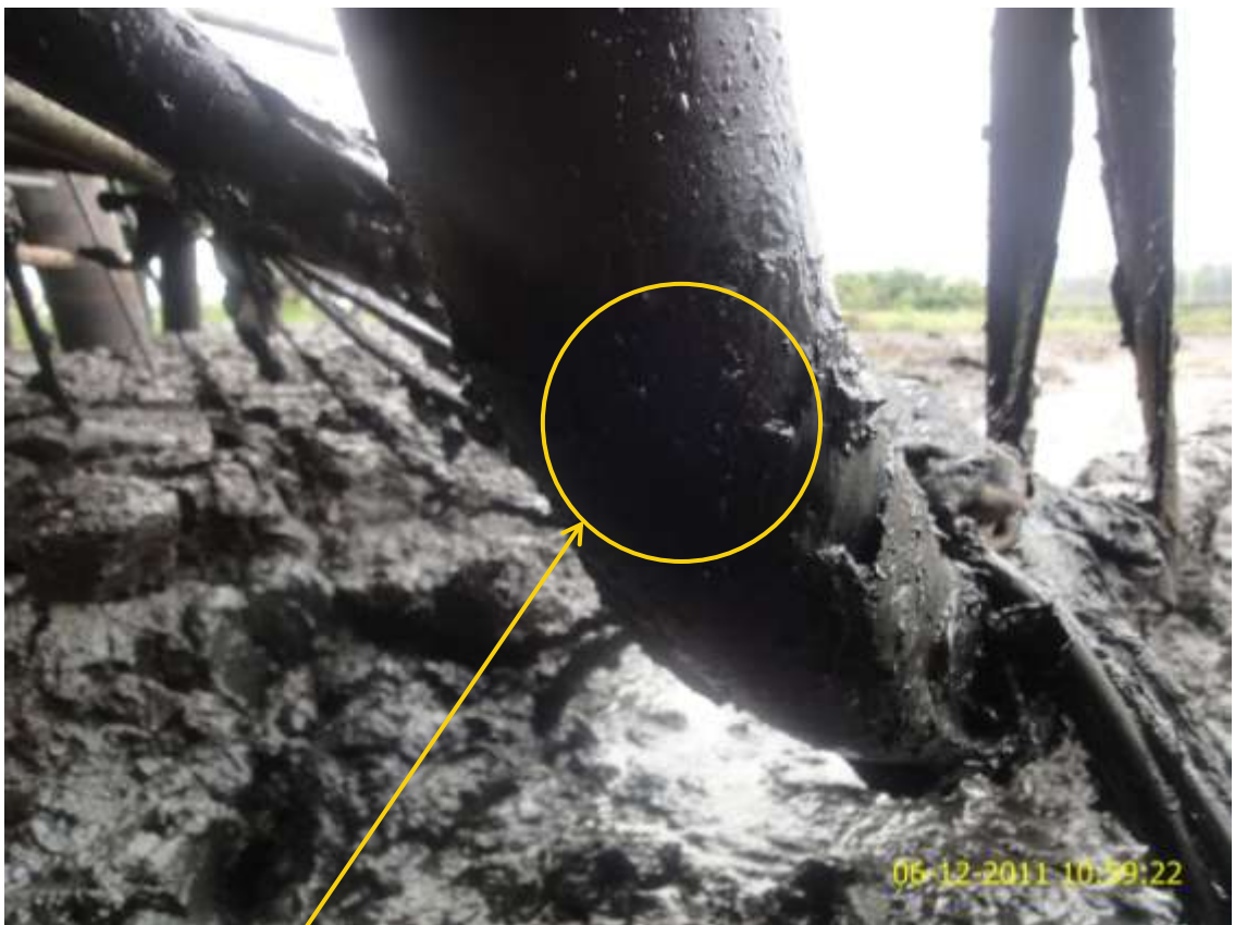
Close-up: Approximate location of pinhole due to corrosion on Awoba Well8T flowline riser at Bille. Picture was taken during Joint Investigation of 6 th December, 2011.
