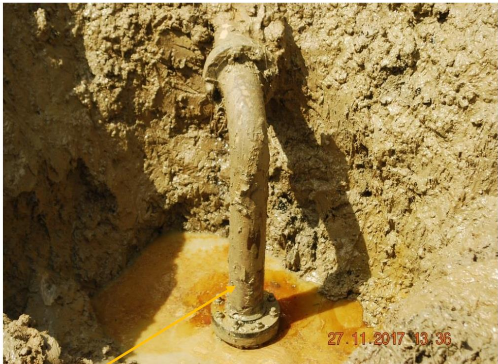
Close-up: Illegal fitting on 20"Kolocreek-Rumuekpe Pipeline at Odau_Ozochi. Picture was taken during Joint Investigation of 27 th November 2017.
