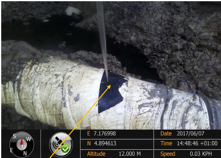
Close-up: Drilled Hole on 12"Imo River-Ogale Pipeline at Uzuaku. Picture was taken during Joint Investigation of 7 th June 2017.
