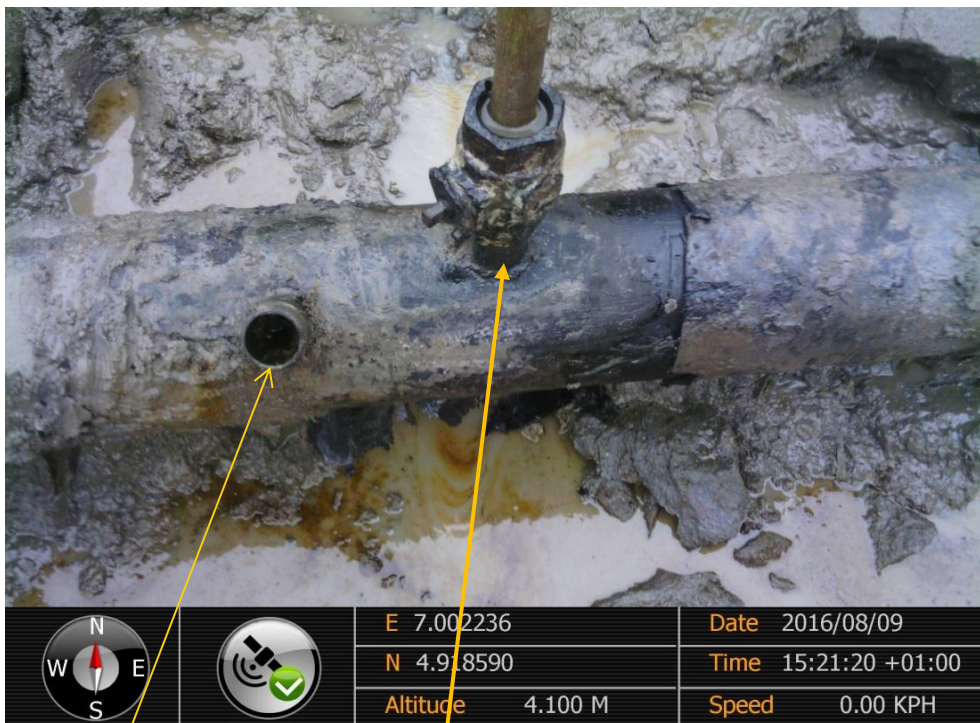
Close-up: Non leaking Illegal point & leaking Illegal fitting on 8" Agbada2-Nkpoku Pipeline at Rukpokwu. Picture was taken during Joint Investigation of 9 th August 2016.
