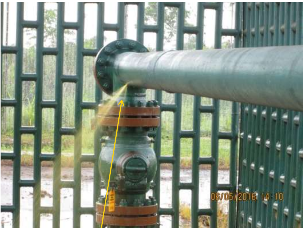
Close-up: Leak point on Ibaa manifold 8" Header at Ibaa. Picture was taken during Joint Investigation of 6 th May 2016.
