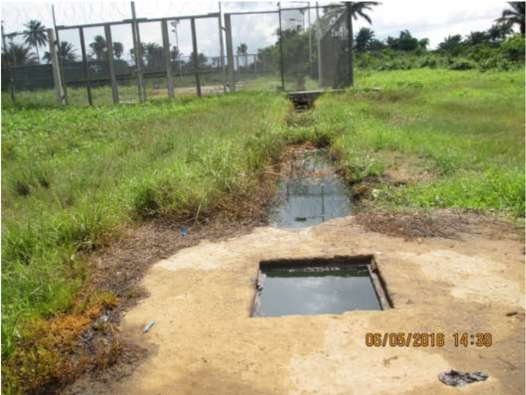
Overview: Part of Spill Impact around Ibaa manifold 8" Header at Ibaa. Picture was taken during Joint Investigation of 6 th May 2016.
