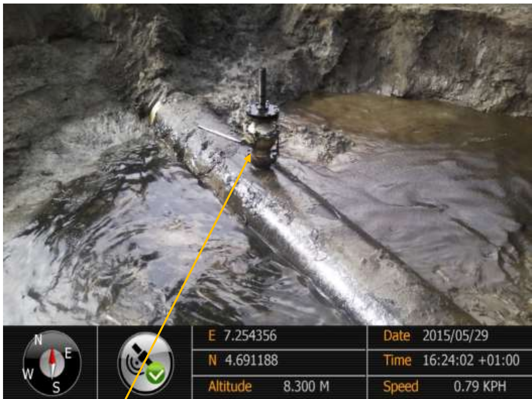
Close-up: Illegal fitting on 28" Nkpoku - Bomu Pipeline at B-Dere. Picture was taken during Joint Investigation of 29 th May 2015.
