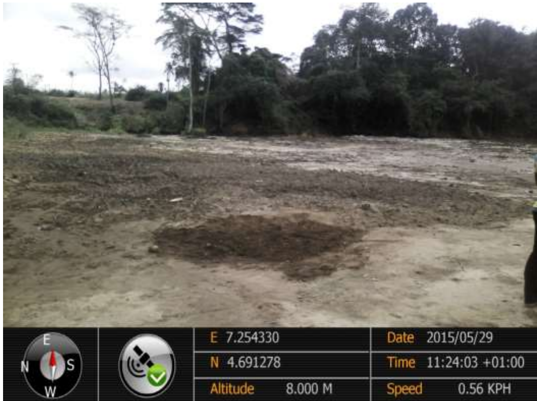
Overview: Part of spill impact on 28" Nkpoku - Bomu Pipeline Right of Way at B-Dere. Picture was taken during Joint Investigation of 29 th May 2015.
