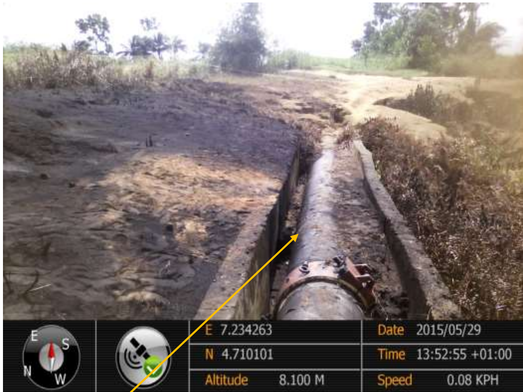
Overview: Location of spill point on 28" Nkpoku-Bomu Pipeline Right of Way at Kpoghor. Picture was taken during Joint Investigation of 29 th May 2015.
