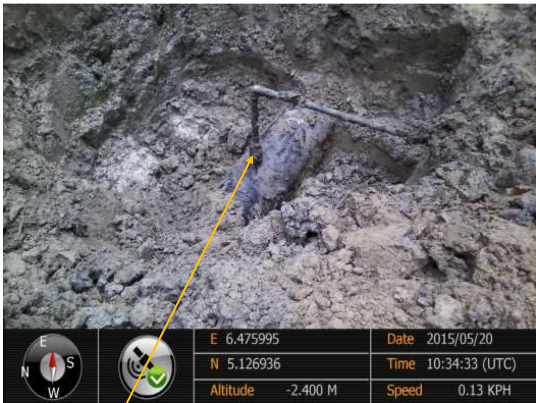
Close-up: Illegal fitting on 14" Okordia – Rumuekpe Pipeline at Akinima. Picture was taken during Joint Investigation of 20 th May 2015.
