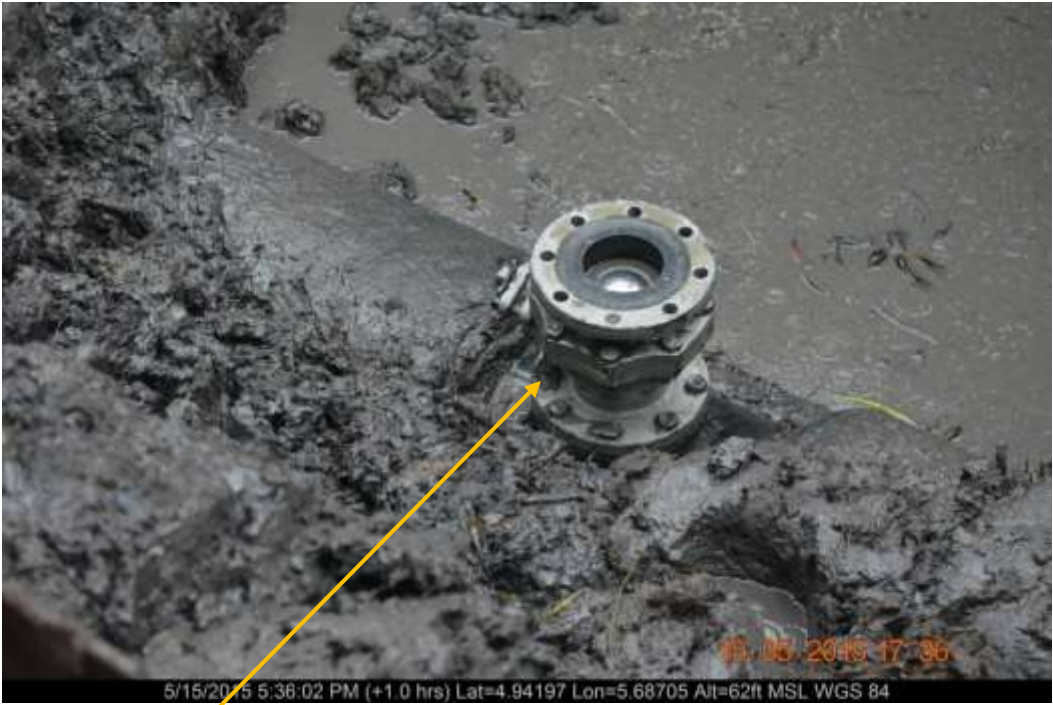
Close-up: Illegal fitting on 20" Opukushi – Brass Creek Pipeline at Tamogbene. Picture was taken during Joint Investigation of 15 th May 2015.
