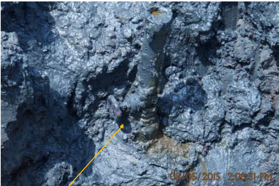
Close-up: Illegal fitting on 20" Otumara-Escravos Pipeline at Ugboegungun. Picture was taken during Joint Investigation of 8 th May 2015.
