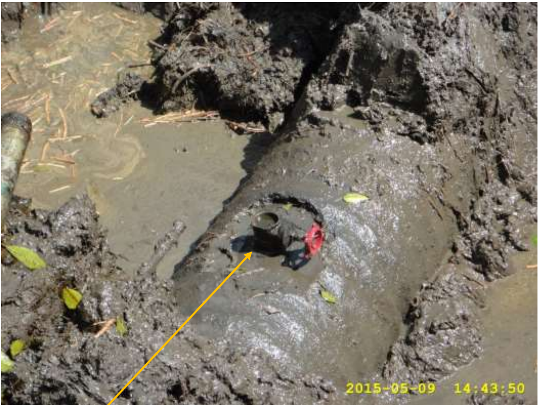
Close-up: Illegal fitting on 28" Bomu-Bonny Trans Niger Pipeline at Otokolomabie/Oloma. Picture was taken during Joint Investigation of 9 th May 2015.
