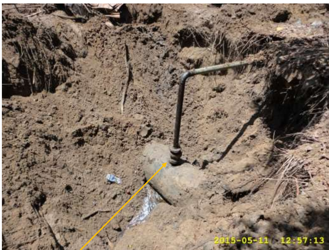
Close-up: Illegal fitting on 28" Bomu-Bonny Trans Niger Pipeline at Otokolomabie/Oloma. Picture was taken during Joint Investigation of 11 th May 2015.
