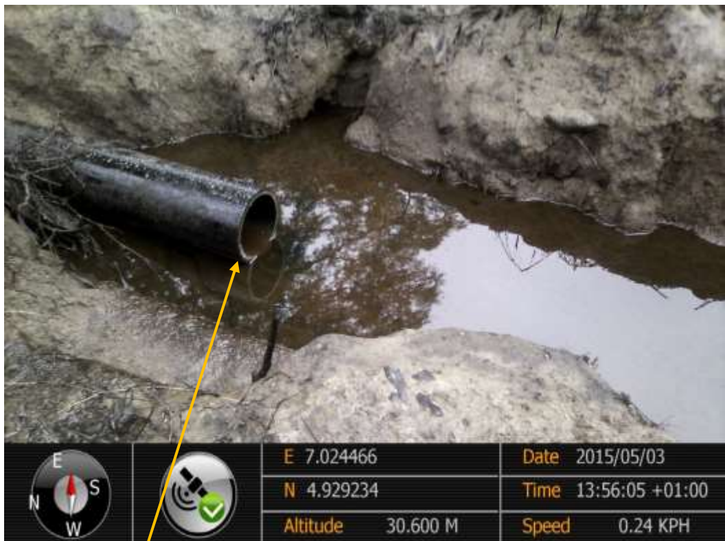
Close-up: Cut section on Agbada 2 Well34S Flowline at Omuohia. Picture was taken during Joint Investigation of 3 rd May 2015.
