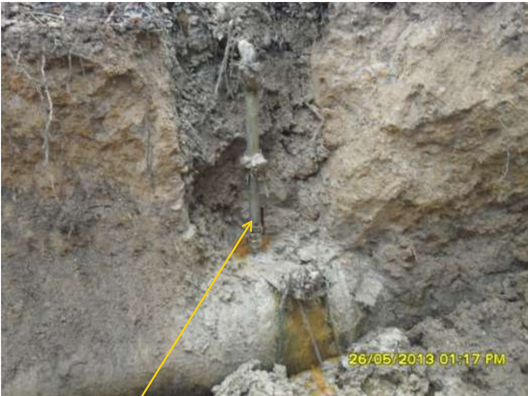
Close up: Illegal fitting on 24" Nkpoku-Bomu pipeline at Egbalor. Picture was taken during Joint Investigation of 26 th May 2013.
