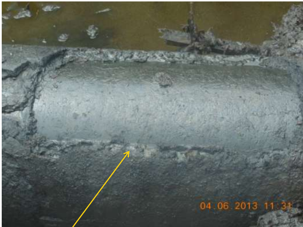
Close up: Section with coating removed on 24" Bomu-Bonny Trans Niger pipeline at BodoWest. Picture was taken during Joint Investigation of 4 th June 2013.
