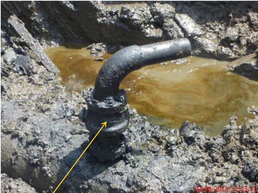
Close up: Illegal fitting on 24" Bomu-Bonny Trans Niger pipeline at BodoWest. Picture was taken during Joint Investigation of 2 nd June 2013.
