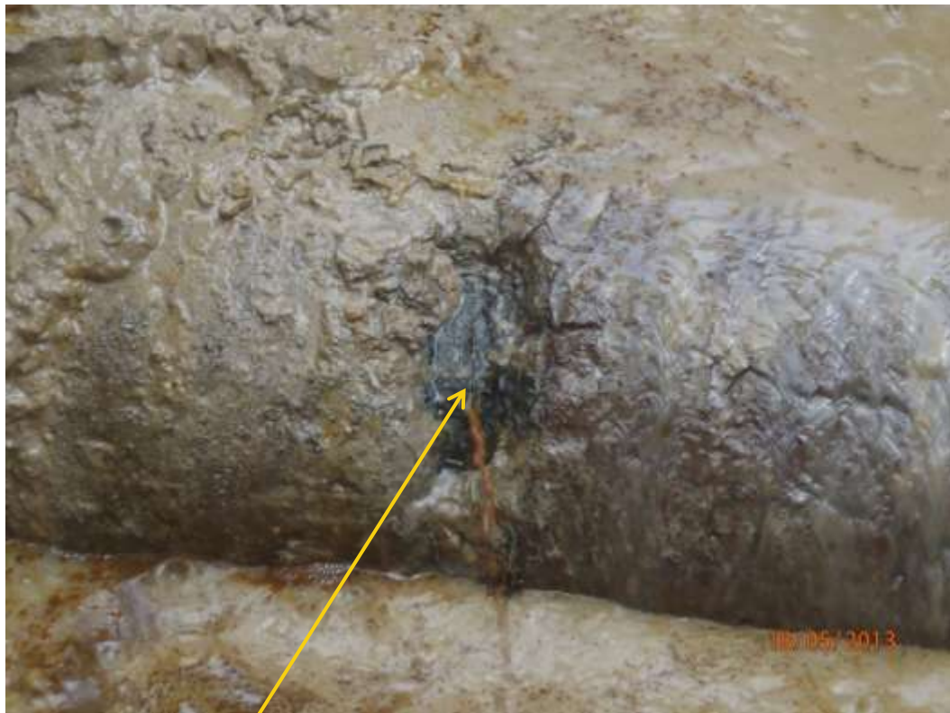
Close up: Spill due to hacksaw cut on 8" Ubie-Ukpeliede pipeline at Idu-Ekpeye. Picture was taken during Joint Investigation of 18 th May 2013.
