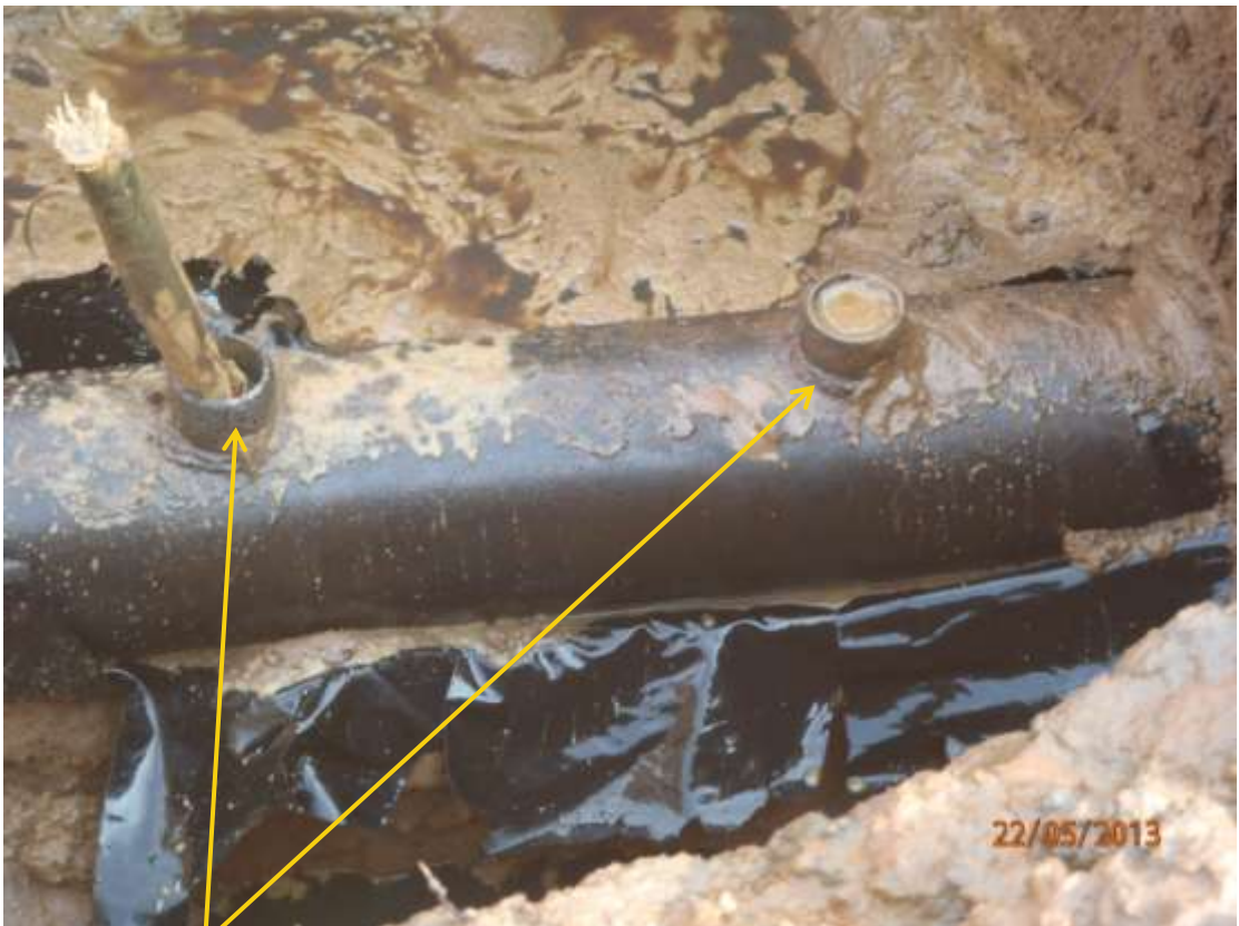
Close up: Illegal fittings on 6" Obigbo North – KomKom pipeline at KomKom. Picture was taken during Joint Investigation of 22 nd May 2013.
