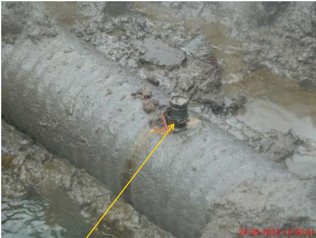
Close up: Illegal fitting on 28" Bomu-Bonny TransNiger pipeline at Bodo West. Picture was taken during Joint Investigation of 24 th May 2013.
