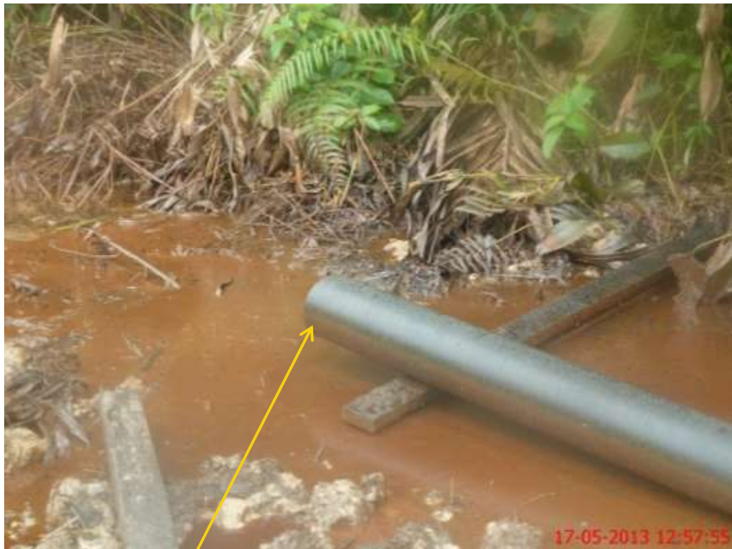
Close up: Cut section of Well20T 6" flowline at Otusega. Picture was taken during Joint Investigation of 17 th May 2013.
