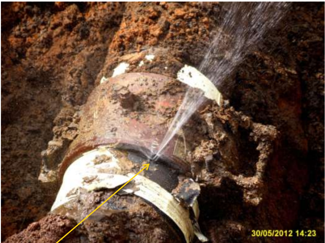
Close up: Hacksaw cut on 18" Assa-Rumuekpe pipeline at Egbeda. Picture was taken during Joint Investigation of 30 th May 2012.
