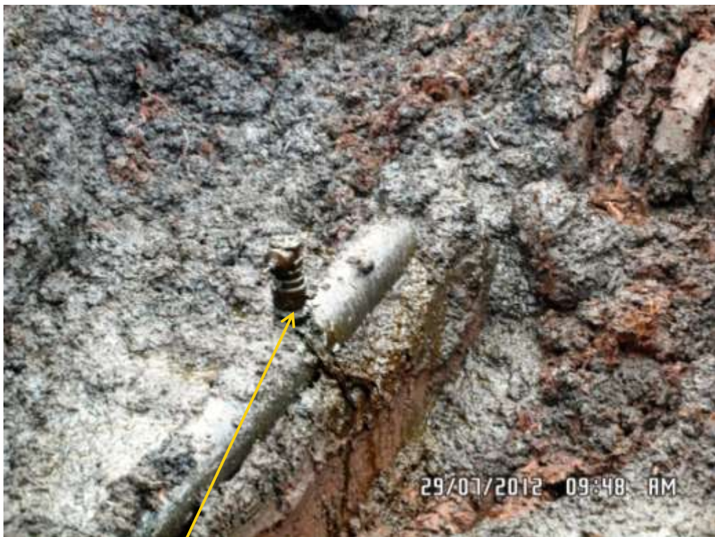
Close up: Illegal fitting on 8" Cawthorne Channel 2 delivery line at Tigerkiri. Picture was taken during Joint Investigation of 29 th July 2012.
