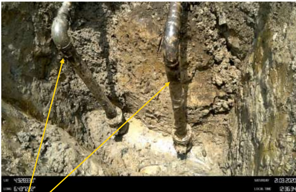
Close-up: Crude oil theft points at 12 o'clock position on Old 20" Kolocreek – Rumuekpe Pipeline at Odau-KP9. Picture was taken during Joint Investigation of 21 st March 2020.
