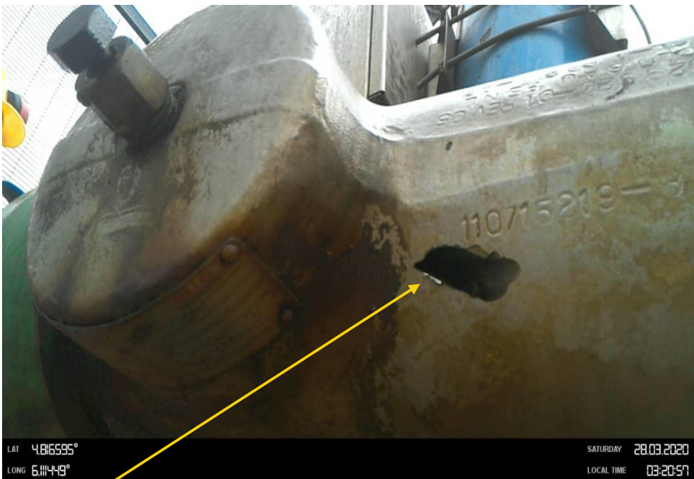
Close-up: Erosion on bean box on NunRiver Well 13T Well head at Angiama. Picture was taken during Joint Investigation of 28 th March 2020.
