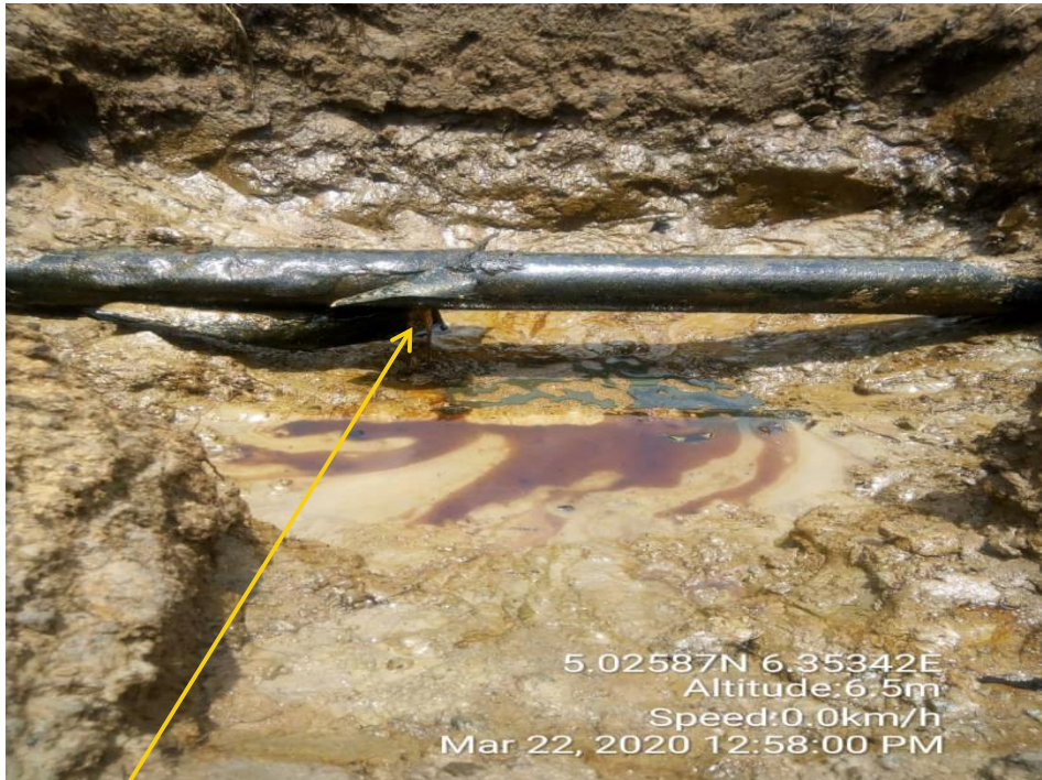
Close-up: Pen size hole at 6 O'clock position on 4" Etelebou Well 1S Flowline at Ogboloma. Picture was taken during Post visit of 22nd March 2020.
