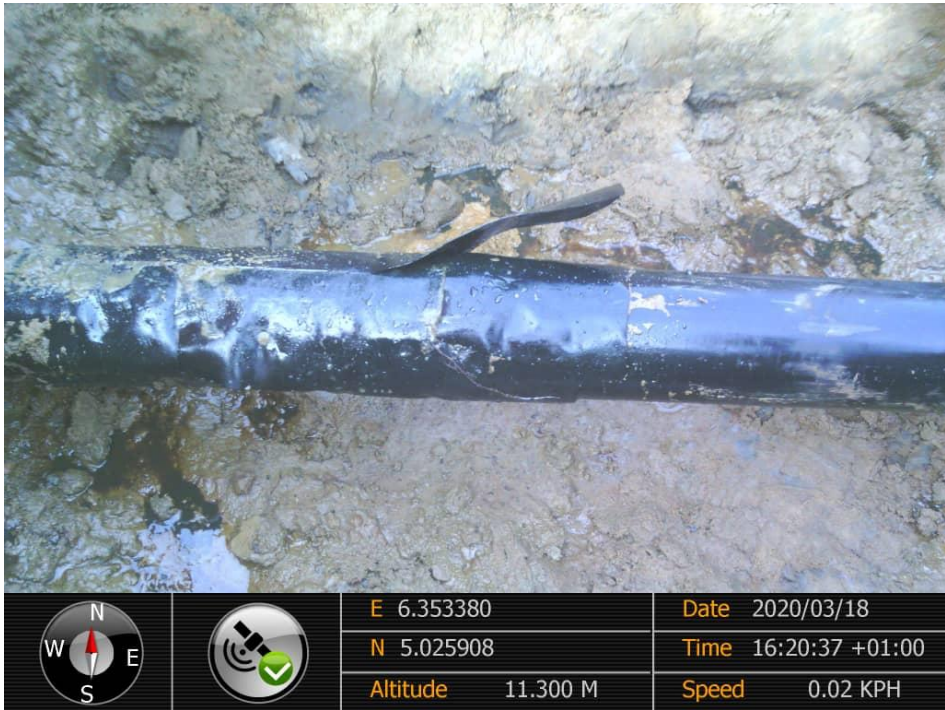
Close-up: 4" Etelebou Well 1S Flowline at Ogboloma. Picture was taken during Joint Investigation of 18 th March 2020.
