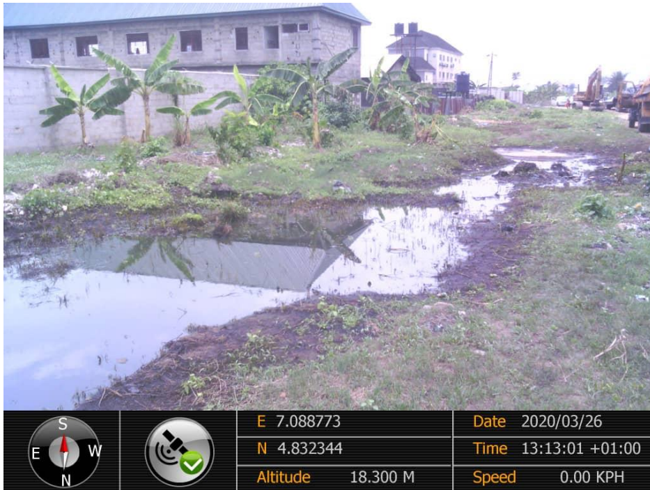
Overview: Part of spill impact on 28'' Nkpoku - bomu Pipeline at Akpajo. Picture was taken during Joint Investigation of 26 th March 2020.
