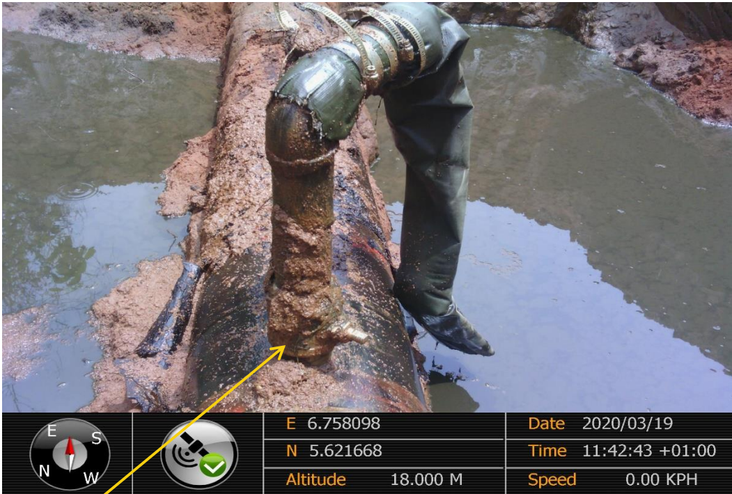
Close-up: 2" valve installed at 12 o'clock position on 12" Oguta – Egbema Pipeline at Eziorsu. Picture was taken during Joint Investigation of 19 th March 2020.
