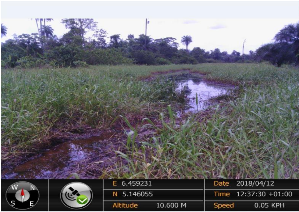
Overview: Part of spill impact on 14" Okordia-Rumuekpe Pipeline at Ikarama. Picture was taken during Joint Investigation of 12 th April 2018.
