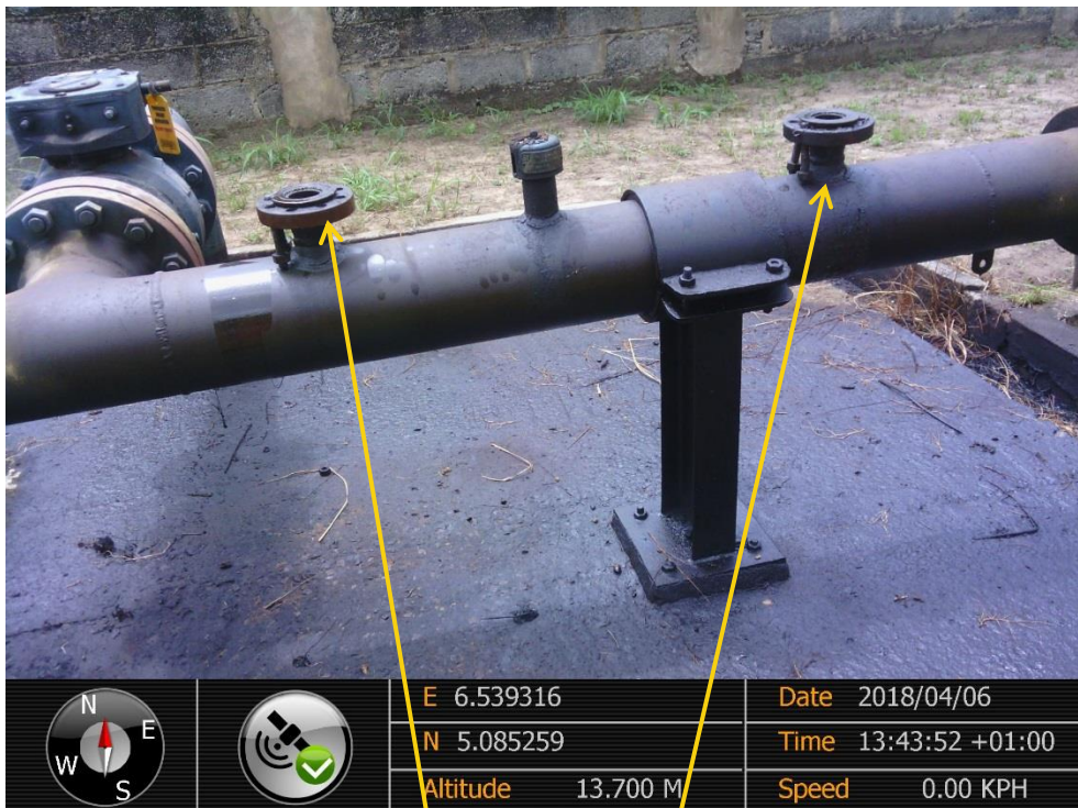
Close-up: Tampered 2" Inlet Pressure Gauge & 2" Inlet Vent Valves on Ukpeliède Manifold at Ukpeliède. Picture was taken during Joint Investigation of 6 th April 2018.
