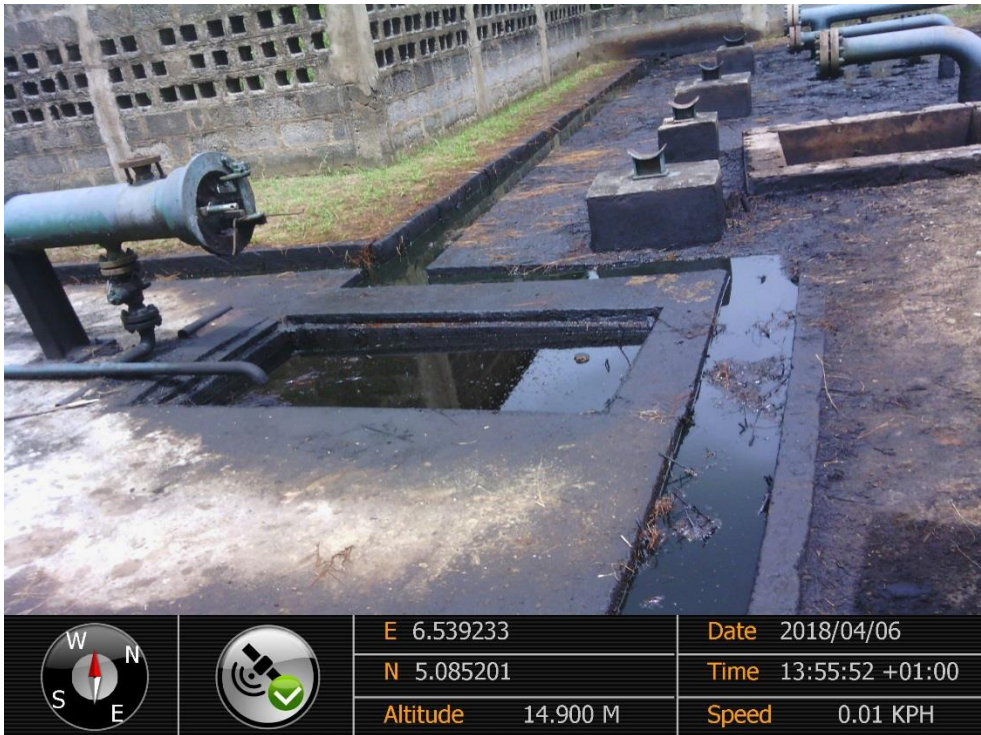
Overview: Part of spill impact on Ukpeliède Manifold at Ukpeliède. Picture was taken during Joint Investigation of 6 th April 2018.
