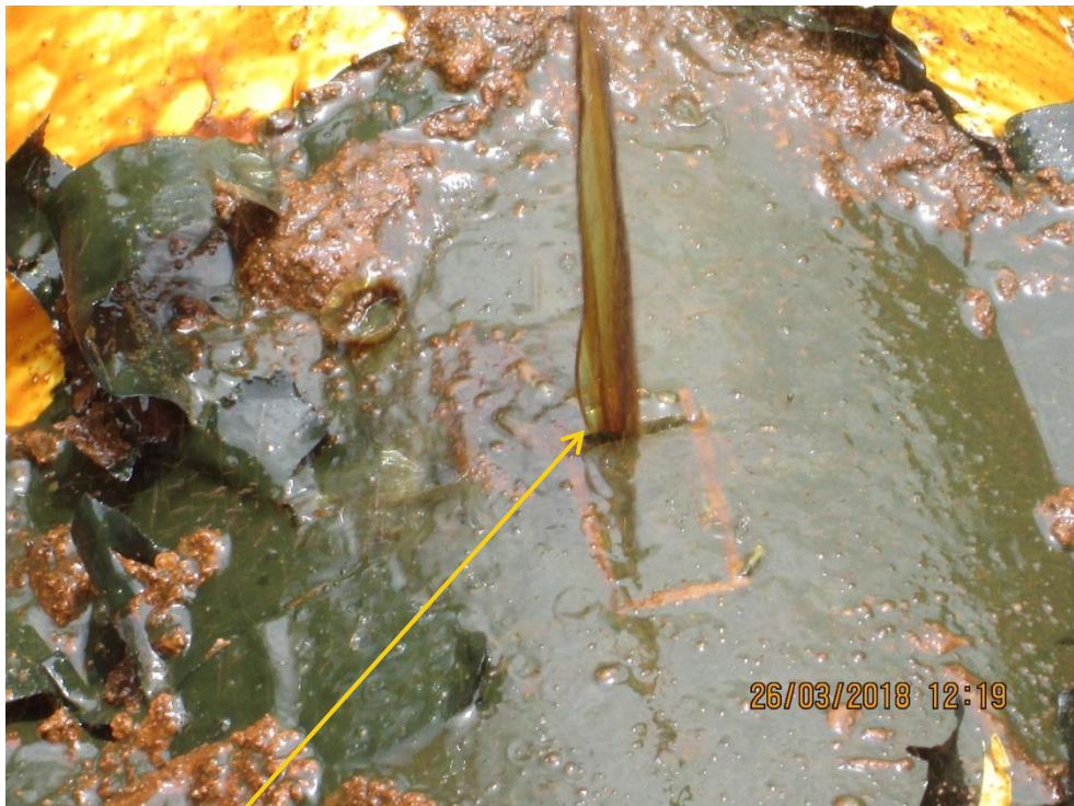
Close-up: Hacksaw Cut on 16" Egbema - Assa Pipeline at Obile . Picture was taken during Joint Investigation of 26 th March 2018.
