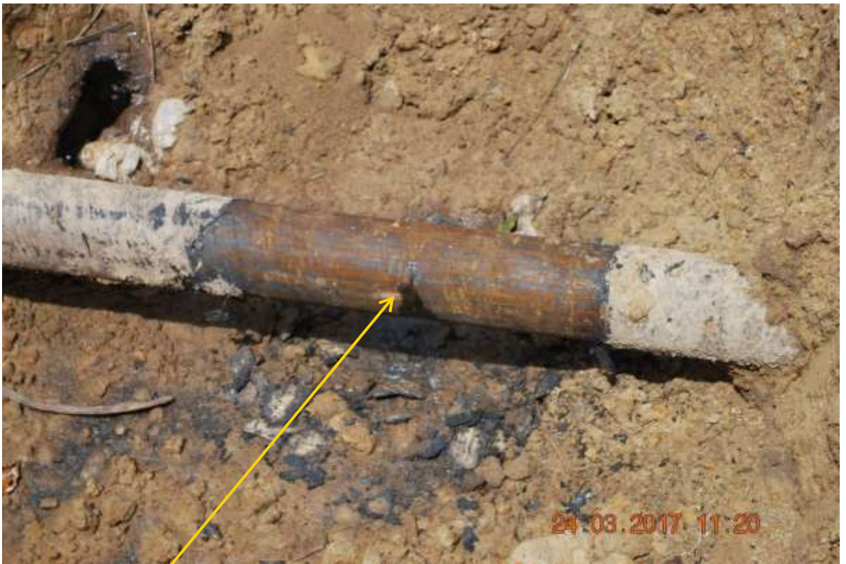
Close-up: Hacksaw cut on 4" Obele-Ibaa Pipeline at Ibaa. Picture was taken during Pipeline Repair on 24 th March 2017.
